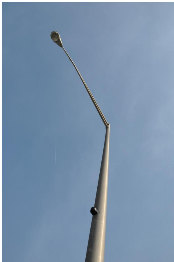
Figure 43: Relay node mounted to light pole
