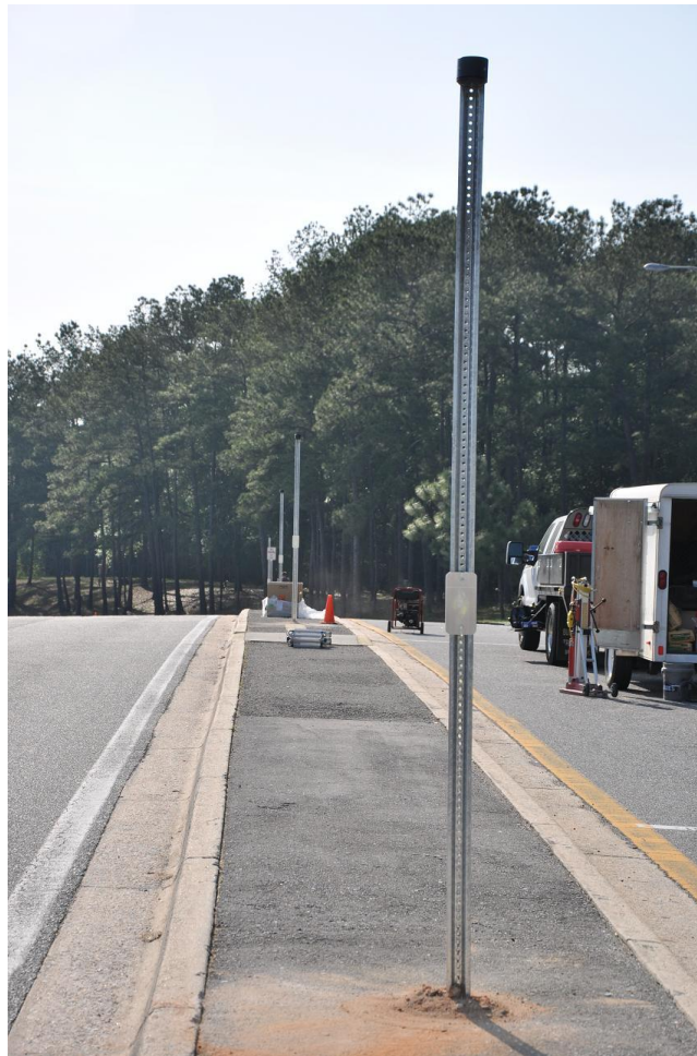
Figure 44: Relay node mounted to traffic sign pole
