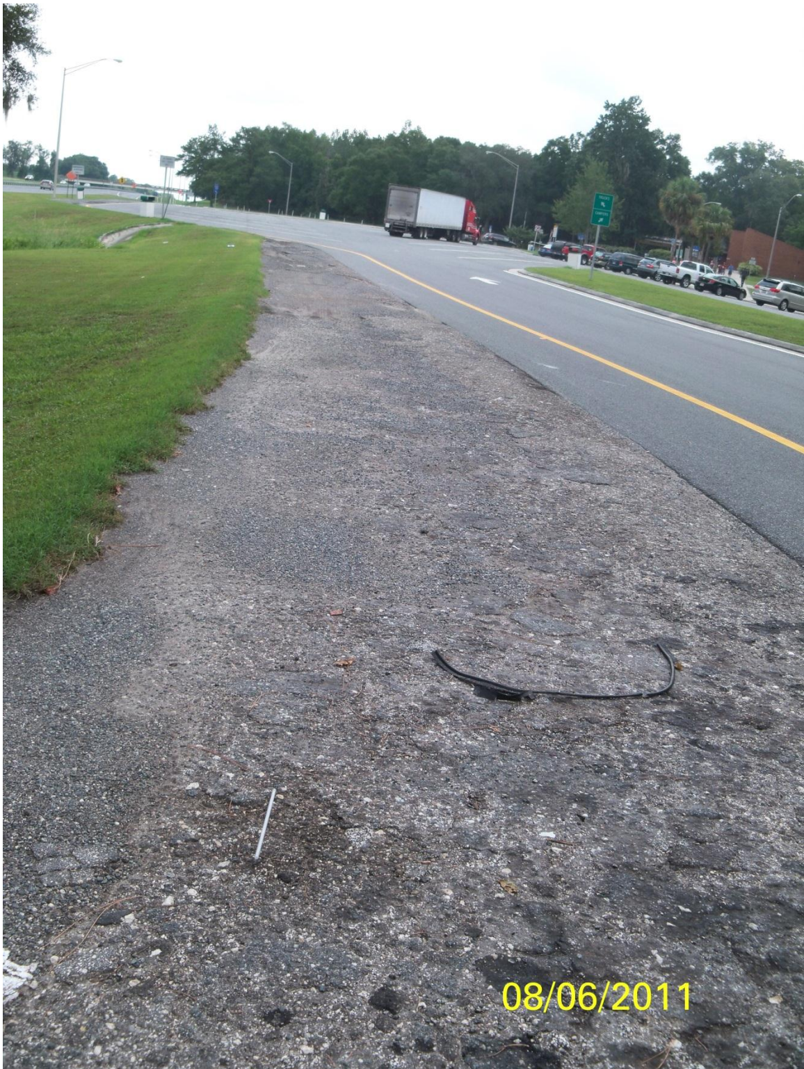
Figure 12: Ruined pavement due to truck parking at Suwannee-Columbia East
